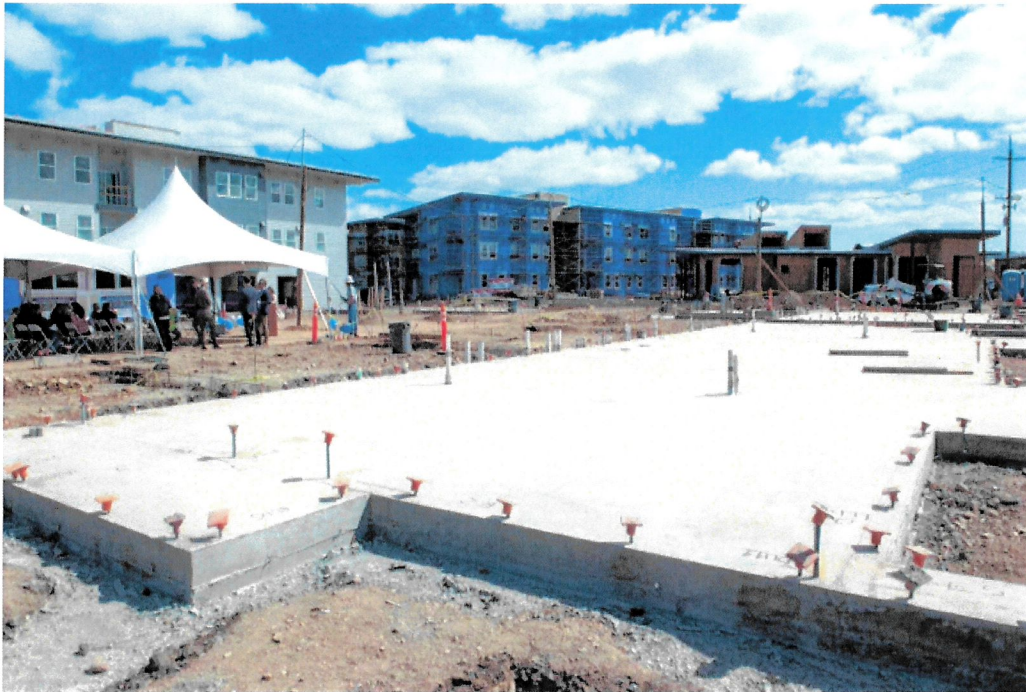
A concrete foundation is seen during a groundbreaking ceremony Friday, June 17, 2022 for the construction of North Creek Crossings in Chico, California. (Michael Weber/Enterprise-Record)
